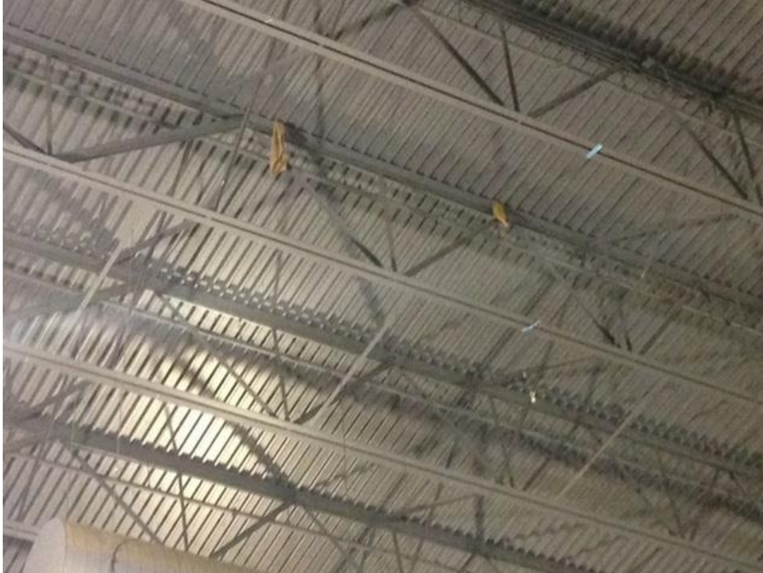
Panel Trusses – located in Halls A, B, C & D – points are rigged where cross bars meet (see where burlap bags are in picture)
